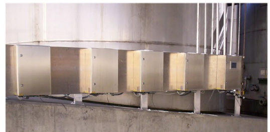
Industrial installation - 120 equipped tanks (California)
